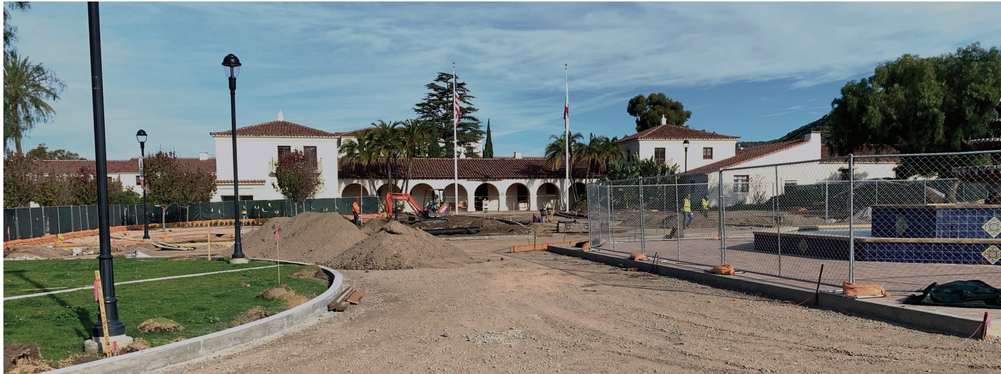
Progress of Central Mall as of Jan. 24. Photo courtesy of Andrew Doran.
